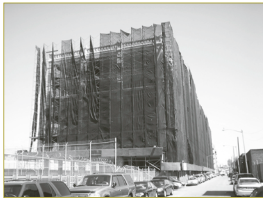
Industrial building at 160 Imlay Street sits vacant in Red Hook. Photo: Kevin E. Schultz.
