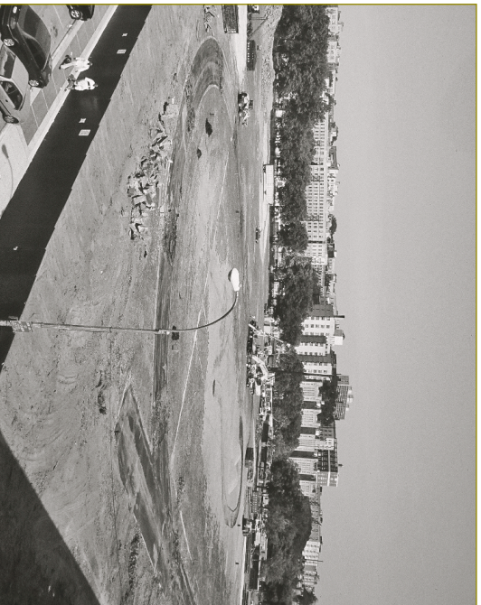
Macombs Dam Park four days after development began on the new Yankee Stadium project. See full story on page 173. Photo: © Geoffrey Croft/NYC Park Advocates. All Rights reserved.
